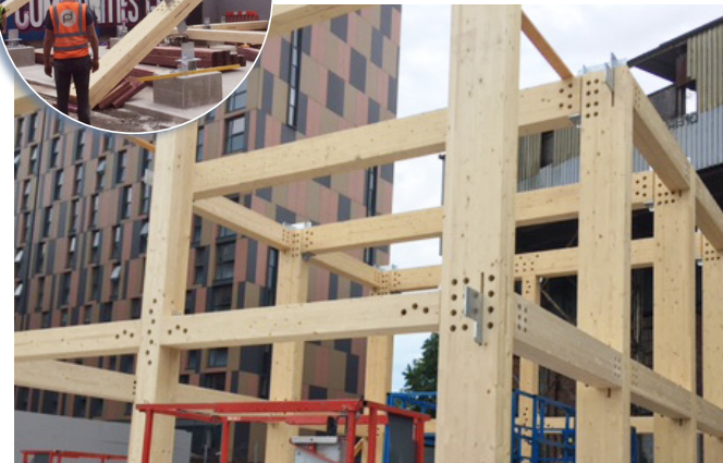
Assembled parts lifted into place, then early stage building commences—with two more storeys to go.
